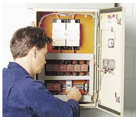
2 C-Bus four channel relays were used to switch lighting at required thresholds
